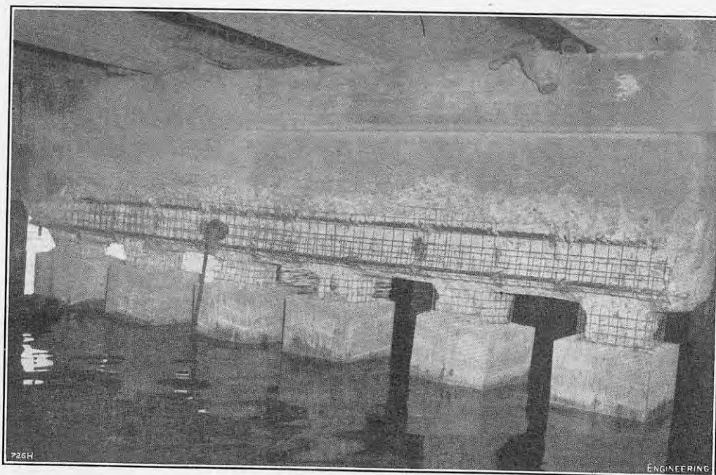
FIG. 8. PILE BENT BEFORE GUNITING.
