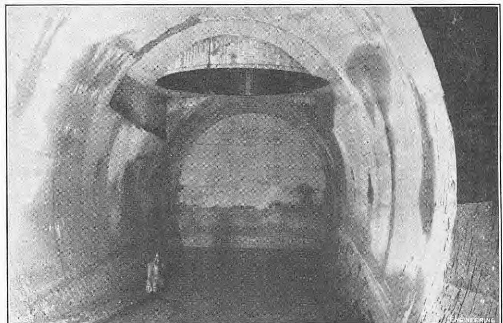
FIG. 5. END OF DISCHARGE TUBE AND DRAUGHT TUBE, MULLARDOCH GENERATING STATION.
