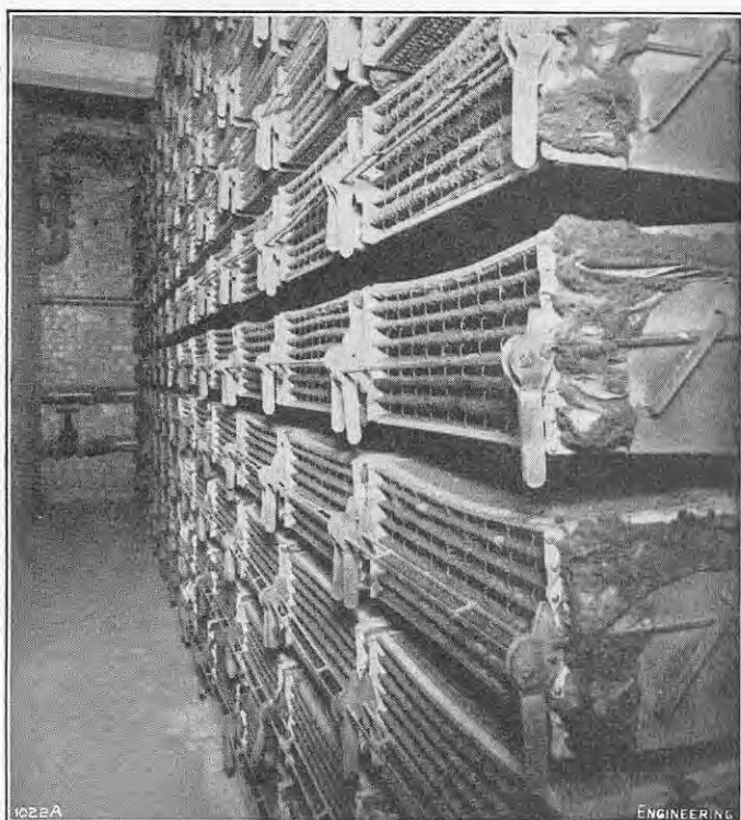
FIG. 1. INLET SIDE OF AIR FILTERS.
