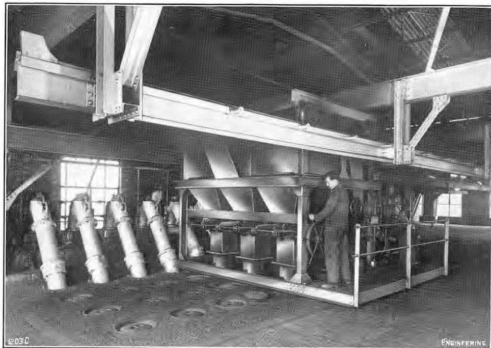
FIG. 3. CHARGING FLOOR AND COAL AND PAD-COKE CHARGING CAR.
