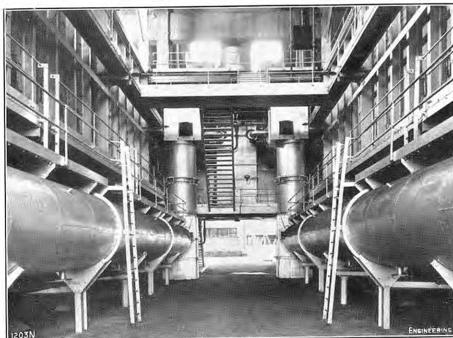
FIG. 14. PRODUCER-GAS MAINS BEHIND BENCHES.
