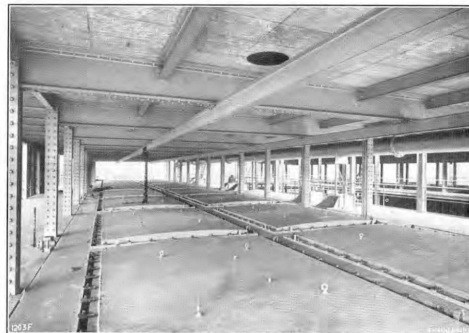
FIG. 6. TOP OF PURIFICATION BOXES.
