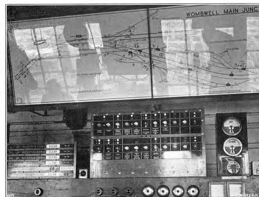
FIG. 13. KEY-SWITCH PANEL AT WOMBELL JUNCTION SIGNALBOX.
