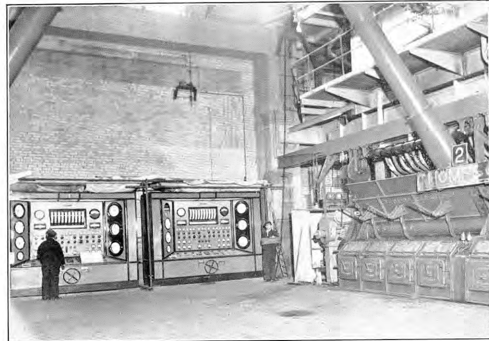
FIG. 3. FIRING FLOOR OF BOILER HOUSE.
