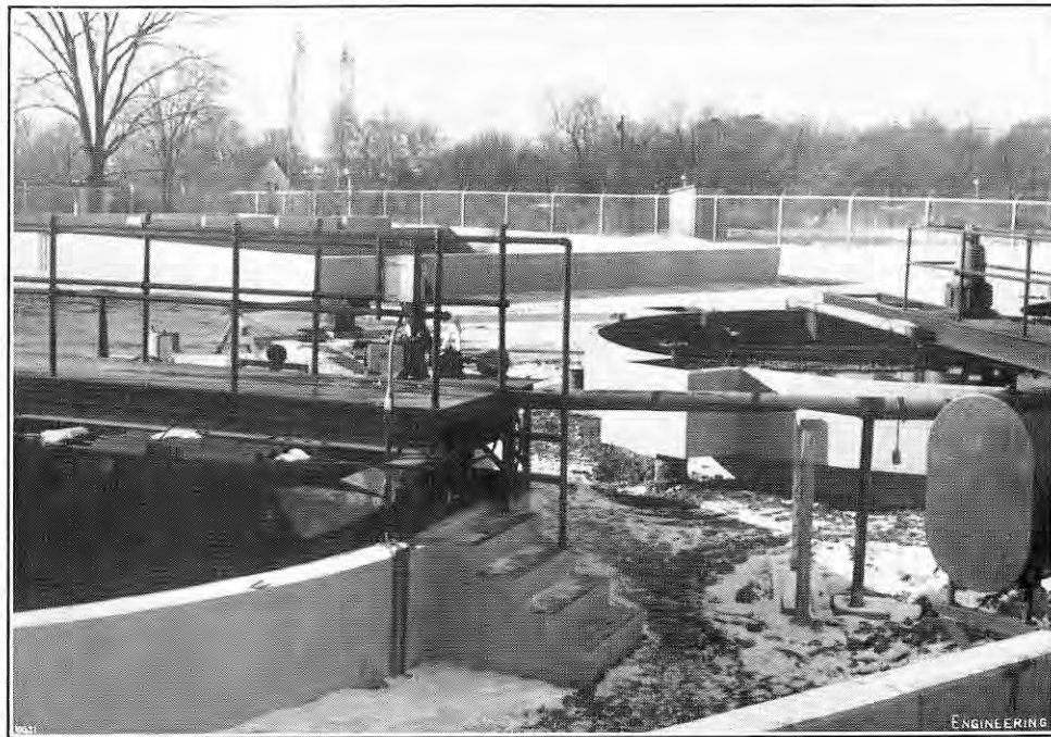
FIG. 11. CYCLATOR AND CLARIFIER.
