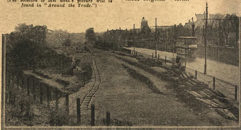
Southern motorists will greatly appreciate improvements which are being carried out on the Uxbridge road. Here is a new section, under construction, alongside Hanwell Asylum.
