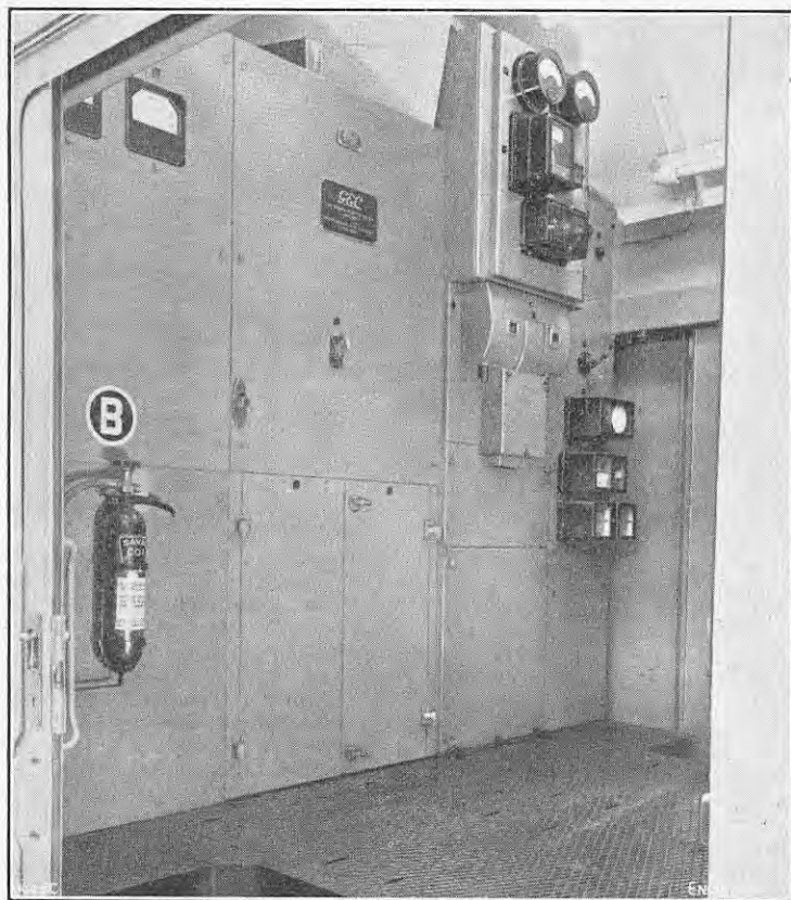
FIG. 3. OPERATING PLATFORM OF MOBILE SUBSTATION.
