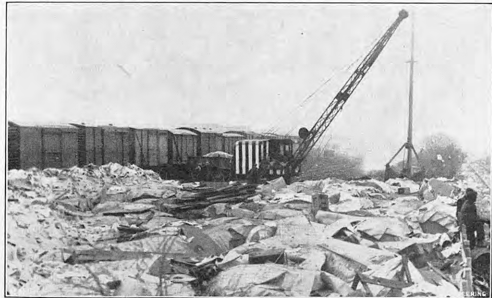
FIG. 4. CLEARING WRECK FROM PURFLEET SIDINGS.
