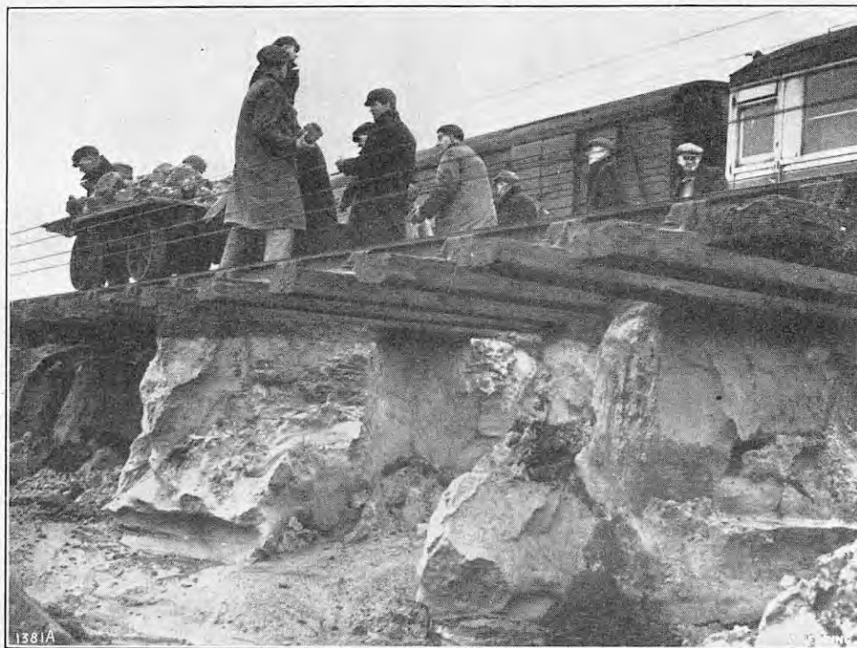
FIG. 1. BREACH IN MAIN-LINE FORMATION.
