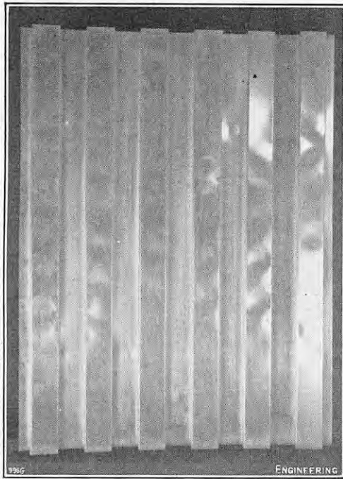
FIG. 7. CORRUGATED PANEL AFTER BUCKLING.
