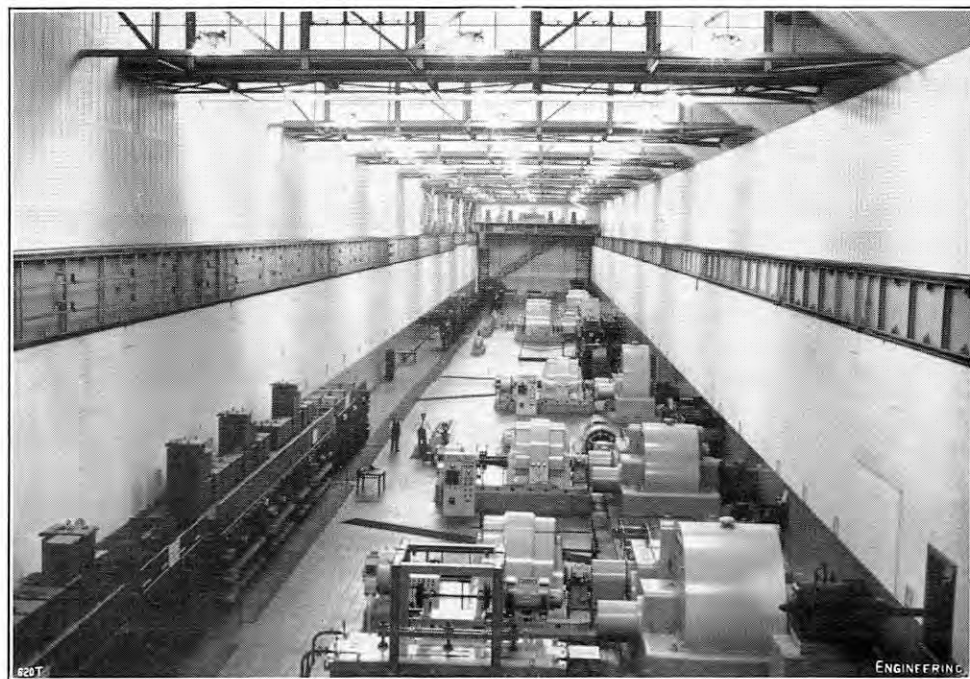
FIG. 19. CONTINUOUS-MILL MOTOR ROOM
