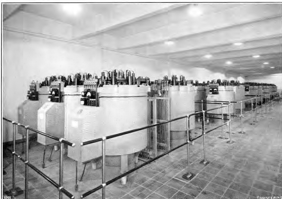
FIG. 21. RECTIFIERS FOR FINISHING STANDS.
