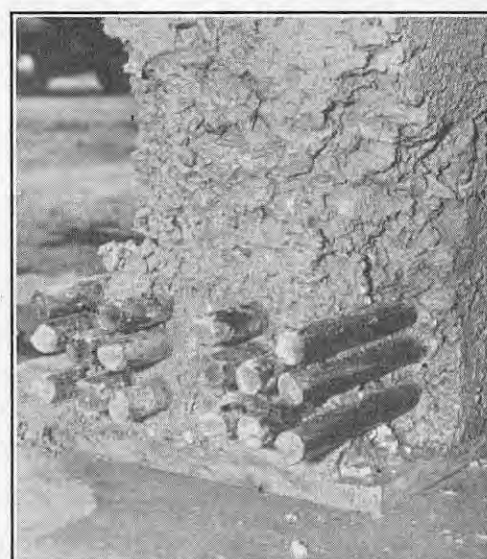
FIG. 13. SHOWING DENSE PACKING OF CONCRETE ABOUT BARS.
