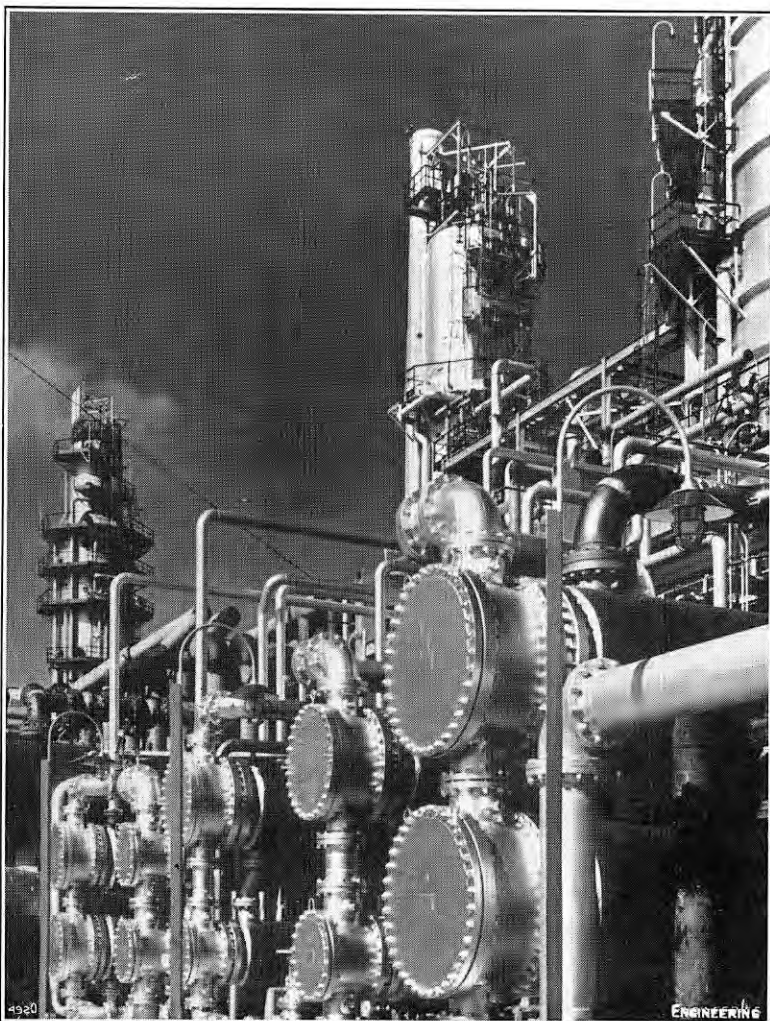
FIG. 9. CRUDE-OIL UNITS WITH HEAT EXCHANGERS IN FOREGROUND.
