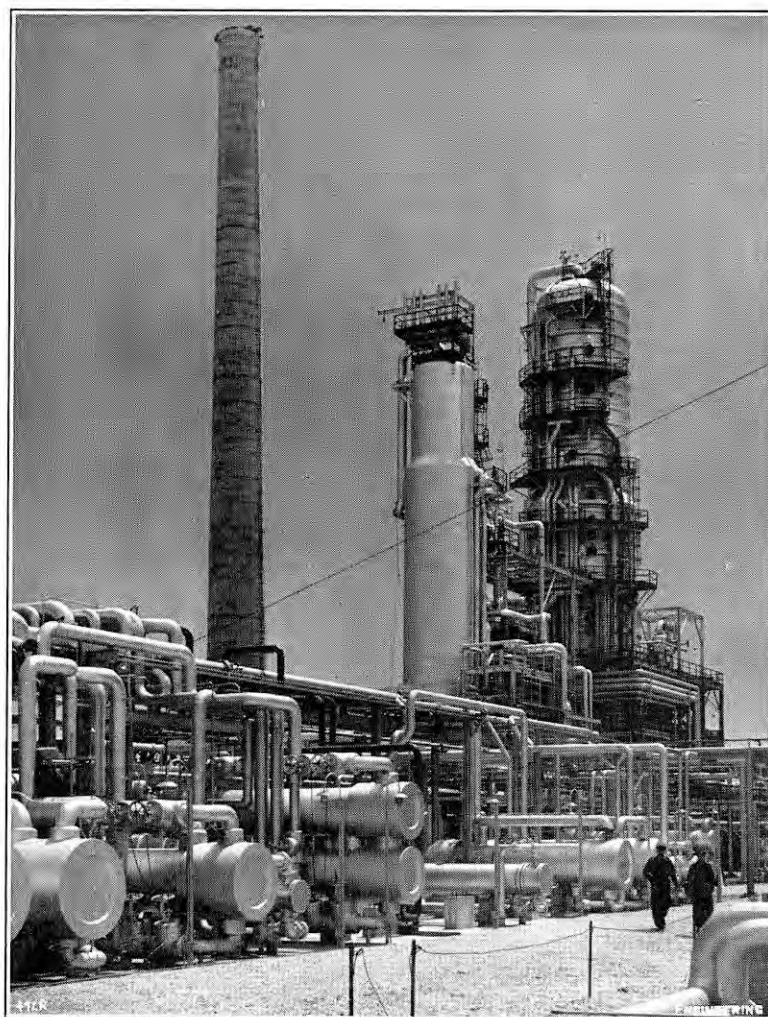
FIG. 12. TWO-STAGE ATMOSPHERIC AND VACUUM UNIT.
