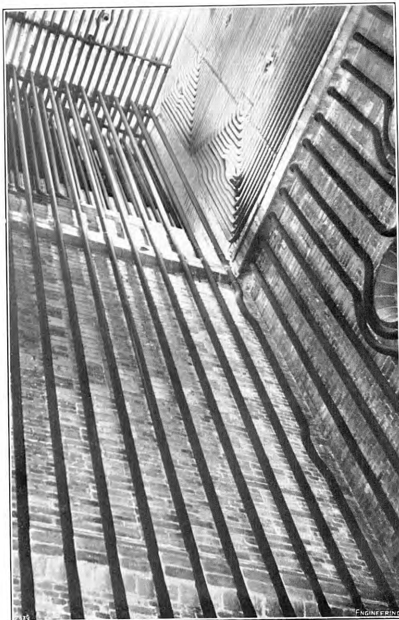
FIG. 7. INTERIOR OF COMBUSTION CHAMBER.
