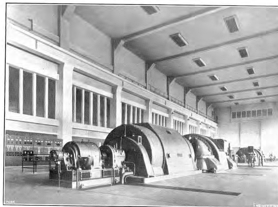
FIG. 13. TURBINE HALL, WITH TWO 50,000-KW TURBO-ALTERNATORS.
