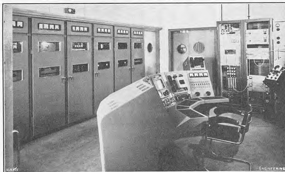
FIG. 2. CONTROL ROOM WITH MEDIUM-POWER TRANSMITTERS.
