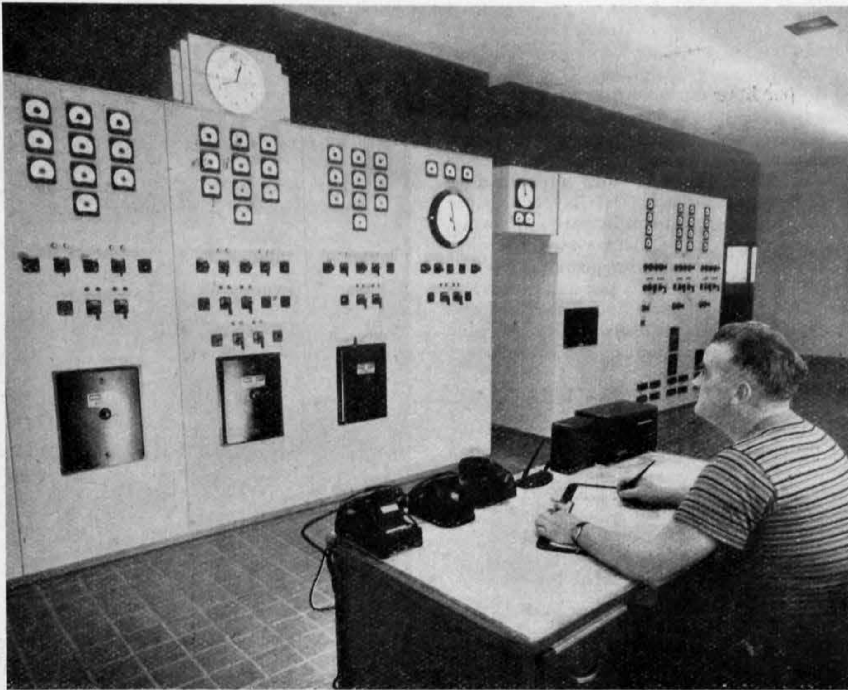
ELECTRICAL CONTROL ROOM
