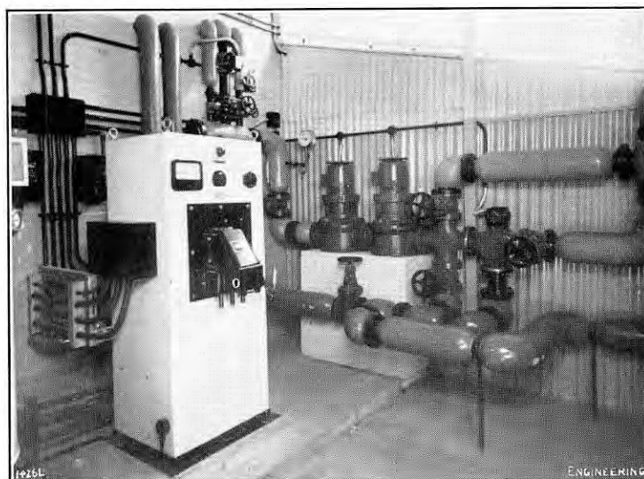
FIG. 11. "AUTOLEC" THERMAL-STORAGE INSTALLATION; G.W.B. ELECTRIC FURNACES, LTD.
