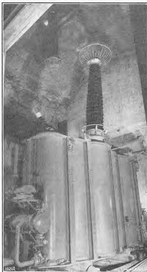
FIG. 1. 115-MVA SINGLE-PHASE TRANSFORMER.
