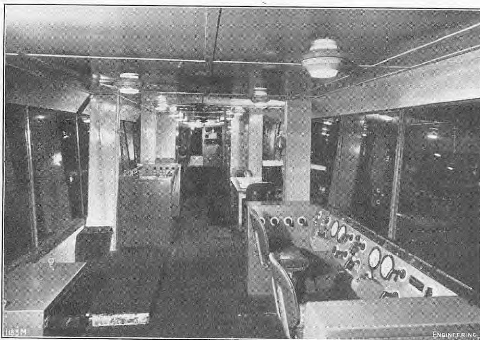
FIG. 14. MAIN CONTROL ROOM.
