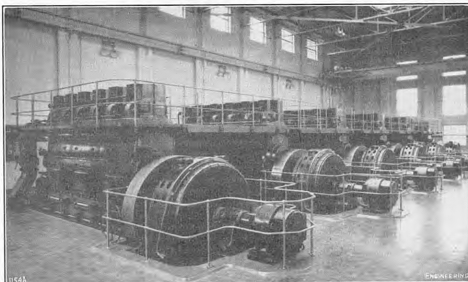
FIG. 1. DIESEL-ENGINE DRIVEN ALTERNATORS.
