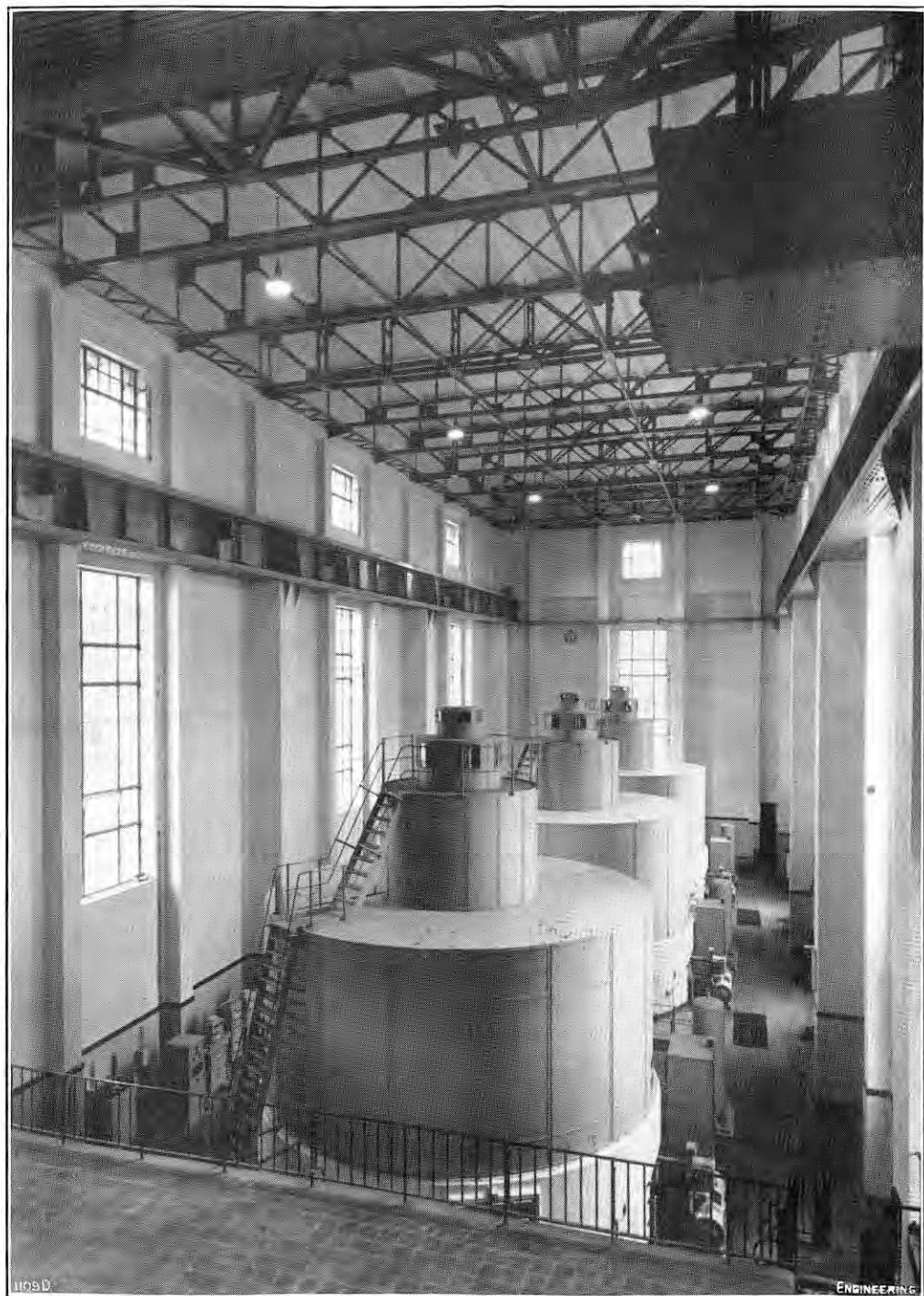
FIG. 40. GENERAL VIEW OF TURBINE ROOM.
