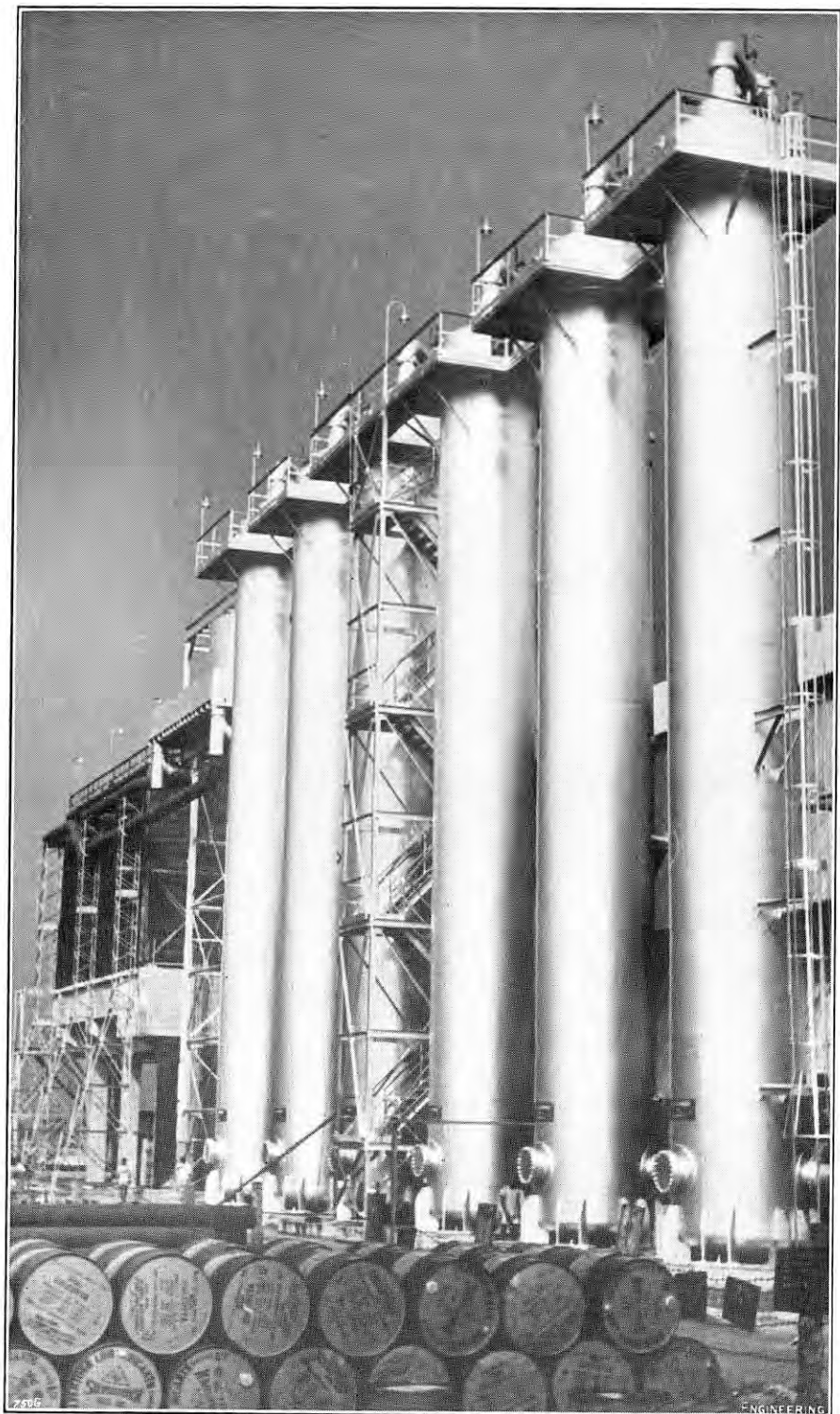
FIG. 7. 75-FT. CARBON DIOXIDE SCRUBBERS.
