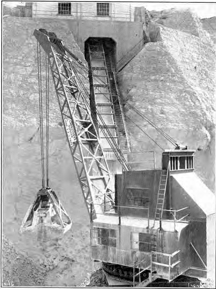
FIG. 8. CHALK CHUTE AND JIB CRANE.
