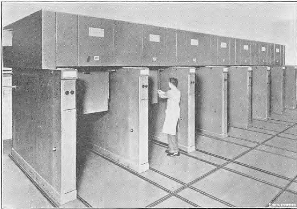
FIG. 66. 1,500-MVA 33-KV METALCLAD SWITCHGEAR; A. REYROLLE AND COMPANY, LIMITED.
